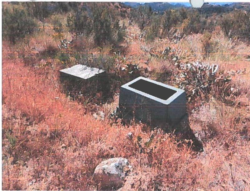
Photograph 1. Electrical conduit was run to the building sites under the previous owner. However, electrical service was never installed.
