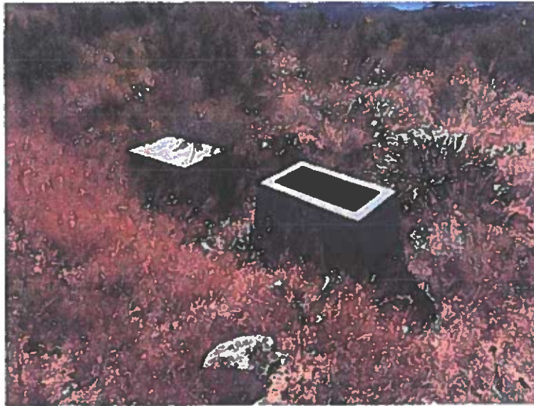
Photograph 1. Electrical conduit was run to the building sites under the previous owner. However, electrical service was never installed.
